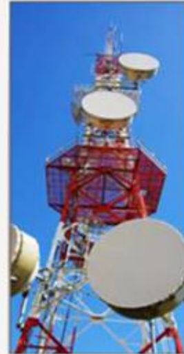
RADIO DEVICES AND TELECOM SHELTER
